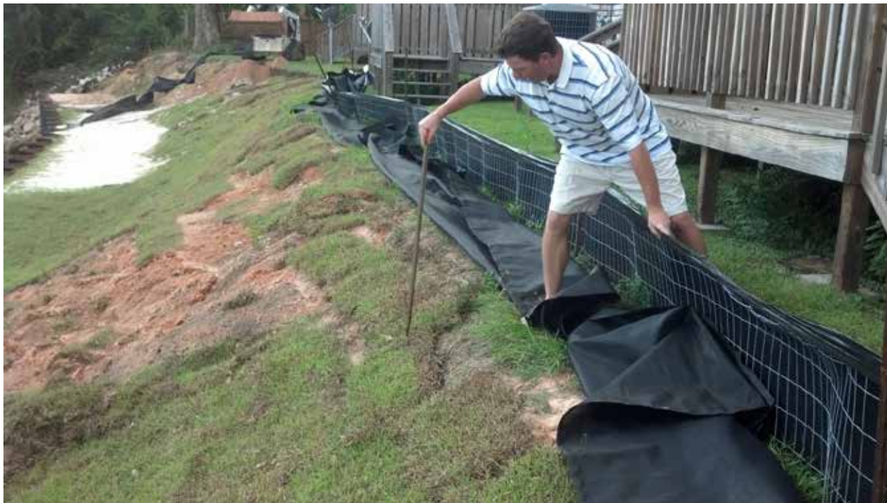
Figure 11. Flooding from the Tchoutacabouffa River caused substantial scouring to the cut bank behind the Rivend Cove Apartments just off Lamey Bridge Rd. A resident (pictured), who stayed during most of the flood event, indicated the high water level to the NWS flood survey team which they used to help estimate the crest for Tchoutacabouffa River at Lamey Bridge Rd (DIBM6).
