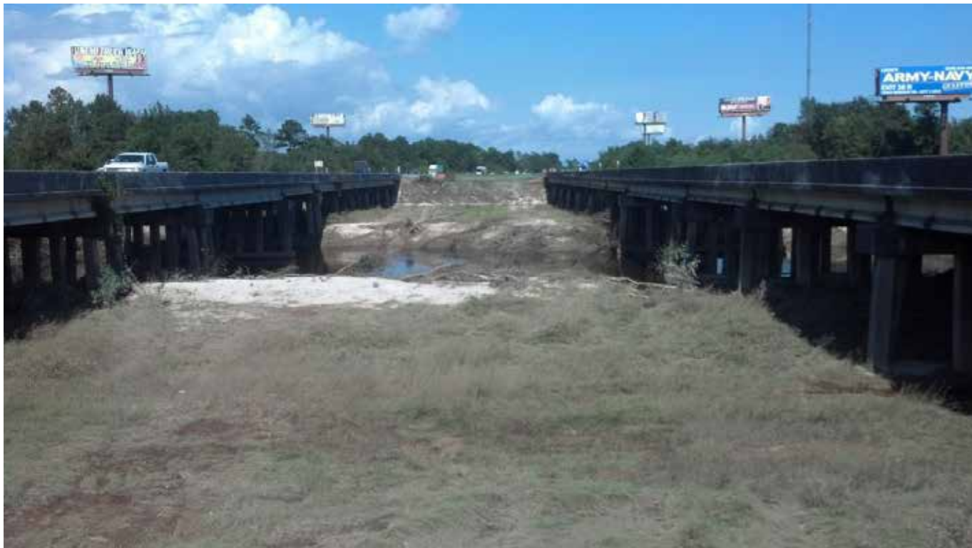
Figure 7. Wolf River floodplain between the eastbound and westbound bridges of I-10. Widespread tree/brush damage was noted along with scouring of the overbank areas.
